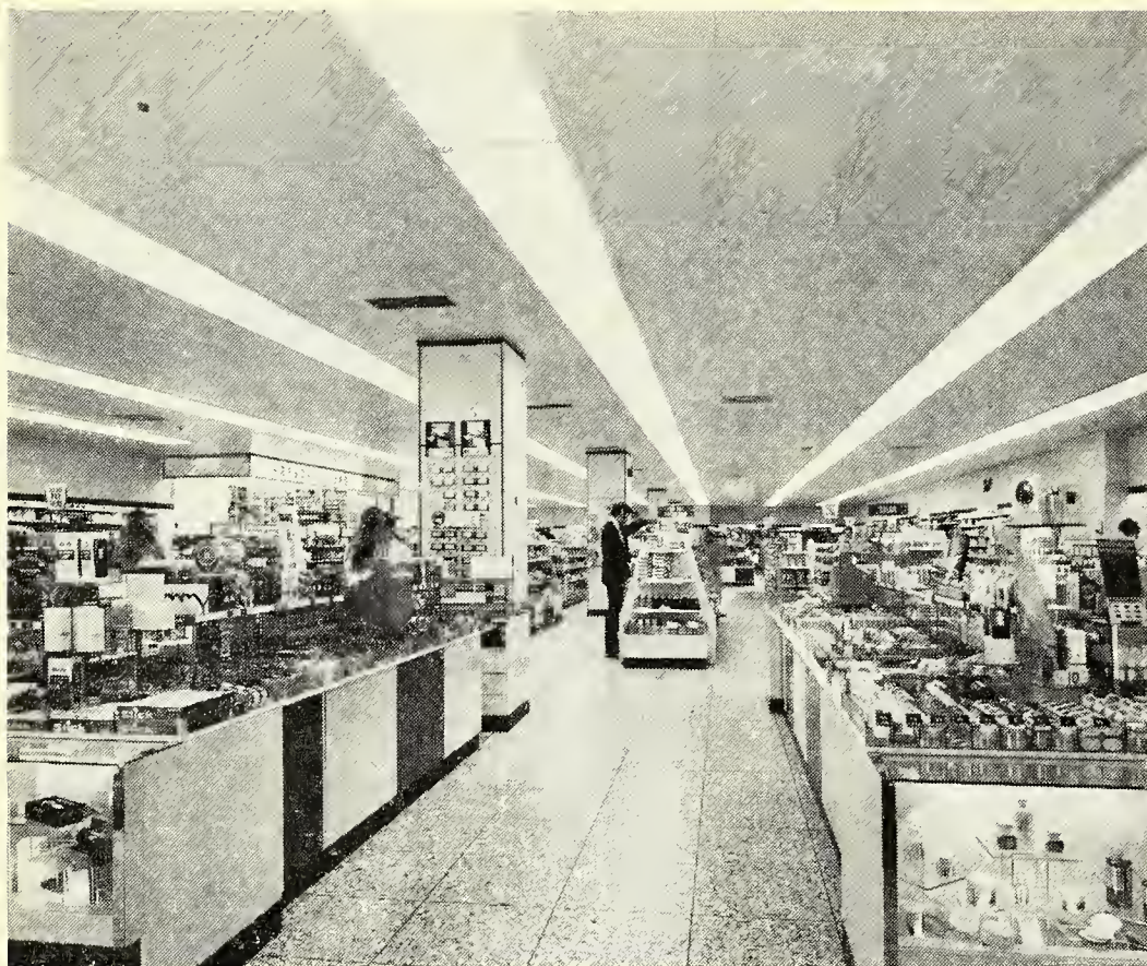
The integrated lighting, heating and air-conditioning system installed at Boots Sunderland store incorporates specially-designed Thorn Lighting fluorescent modular lighting fittings
